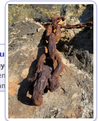
Rusting is a costly form of corrosion
