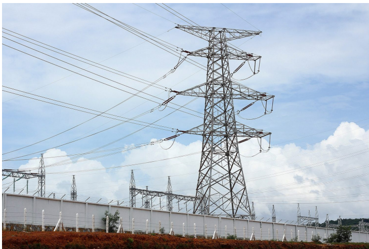
High-voltage power lines: electric potential energy is converted and transmitted as current at high voltage
