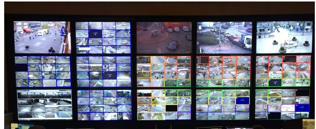
A CCTV control room: surveillance systems trade safety gains against privacy concerns
