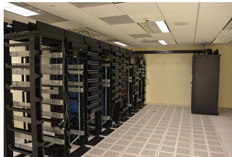
Data-centre server racks: distributed computing spreads work across many machines
