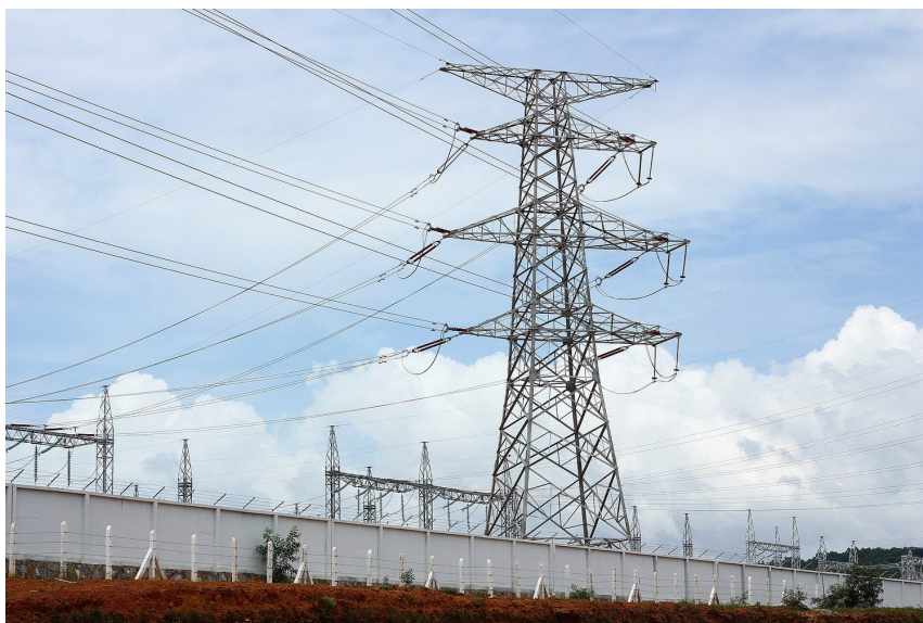
High-voltage power lines carry electrical energy across the country.
